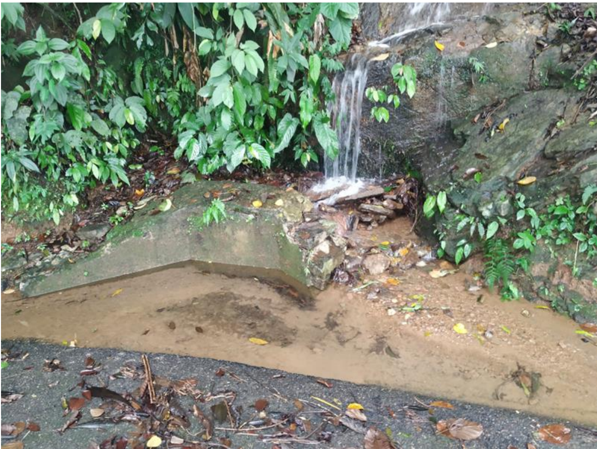
Figure 6 – Manhole completely clogged by sediments coming from a drainage in Central sector. Source: Authors (2022).
