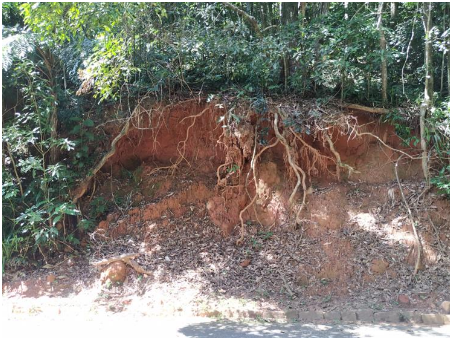
Figure 5 – Road cut in soil with a small mass movement and roots exposure, culminating in the increase of erodibility rate and hazard level. Source: Authors (2022).
