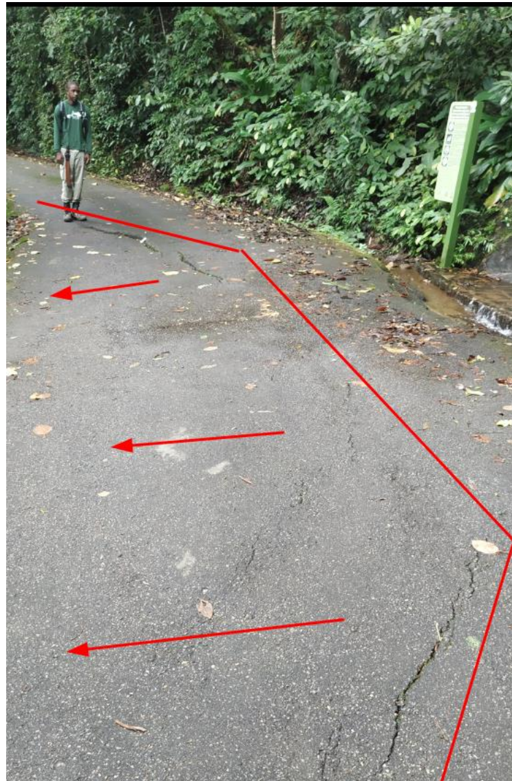
Figure 7 – Road cracks with significant displacement nearby a clogged manhole, indicating subsidence towards downstream. Source: Authors (2022).
